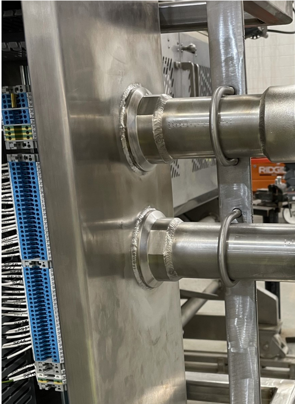
Welded piping system used as a raceway in violation of NEC and OSHA regulations
