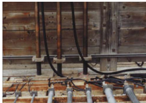
Photo 8. Ten runs of RMC, IMC, and EMT metric designator sizes 16 (1/2 trade size) through 78 (3 trade size) connected to the transformer for high current and low current tests.
