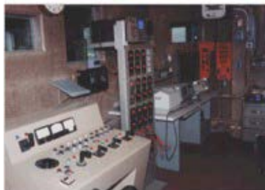
Photos 3 and 4. Kearney Laboratories Outdoor Test Site in McCook, Illinois. This is the large transformer used for the tests and all data was recorded with instruments inside the building. All data was recorded by Kearney's engineering department and Dr. Meliopoulos using separate test instruments. This was done to validate the data.
